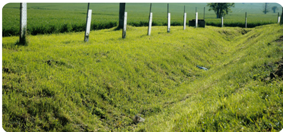
Fig. 2: Grassed retention ditch as designed in the Czech Republic (Dzuráková et al., 2017).
